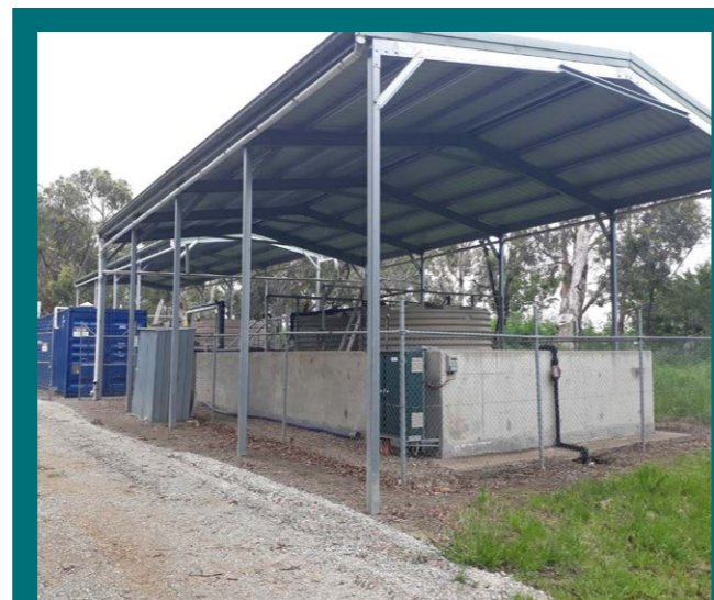
Coldstream leachate plant – the plant processes leachate liquid collected from the landfill for disposal into the sewer system. This is important to ensure that the liquid does not contaminate local groundwater and the surrounding environment.
